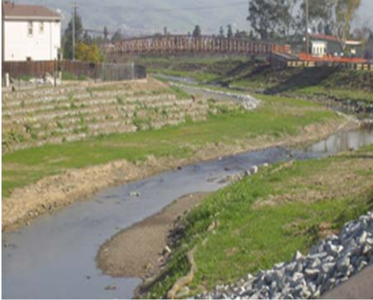
Figure 14: Silver Creek Restoration and Newly Constructed Pedestrian Bridge in the Mayfair Community
