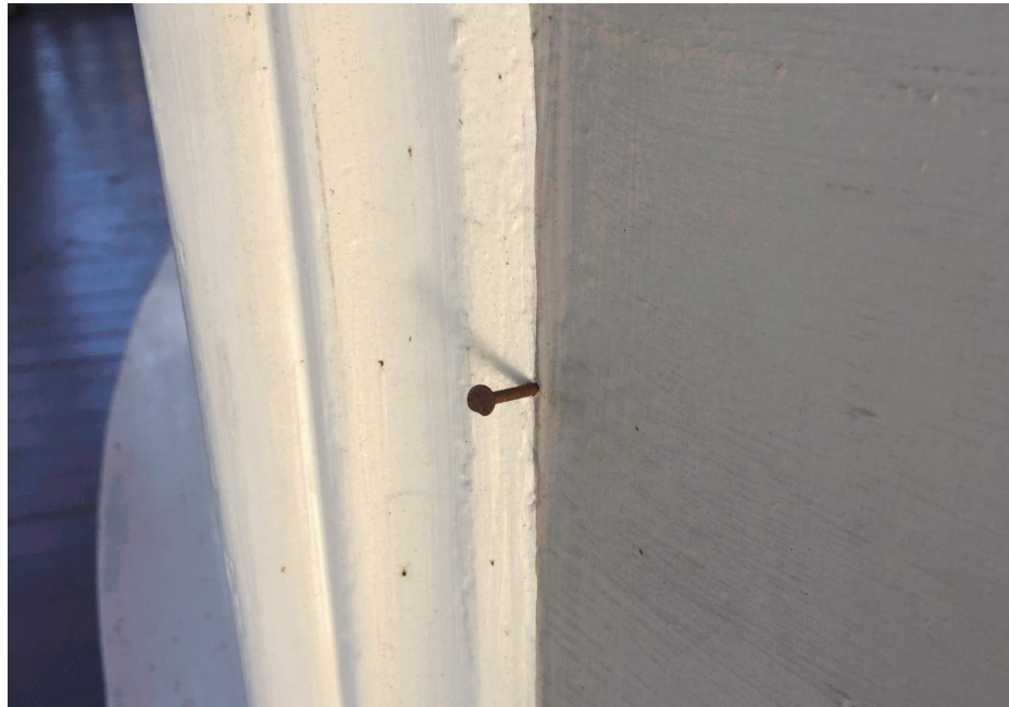
Nails used on the historic exterior should not be mild steel, 2017 (Page & Turnbull)
