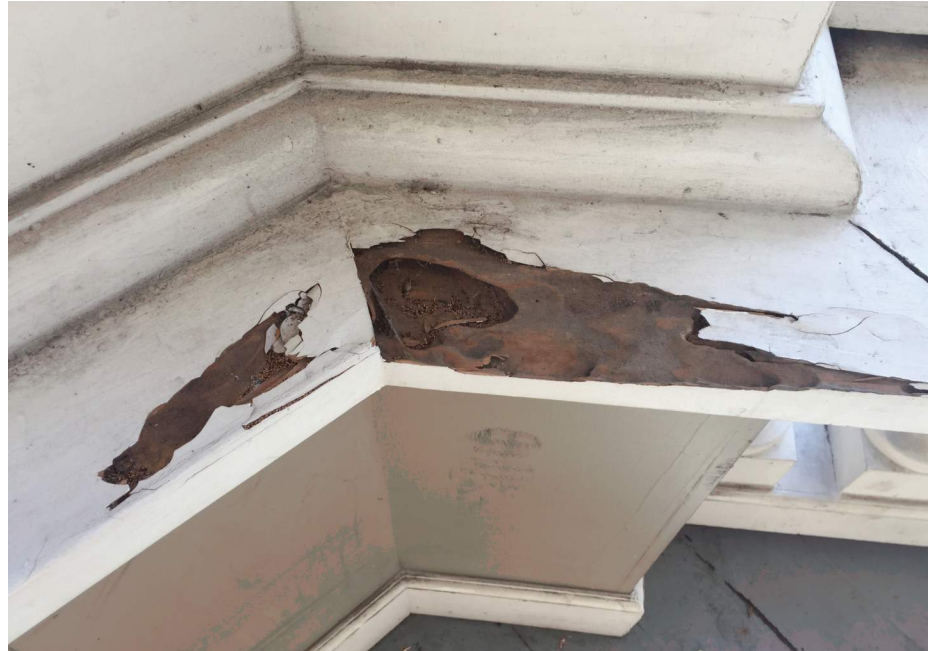
Insect damage in porch railing, 2017 (Page & Turnbull)
