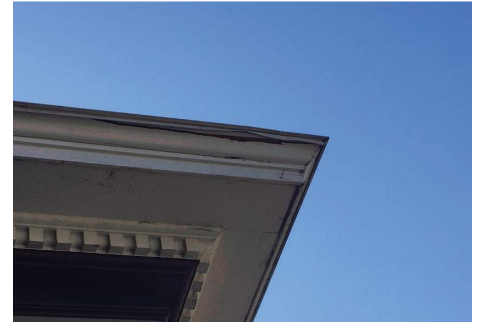
Broken roof edge, 2017 (Page & Turnbull)
