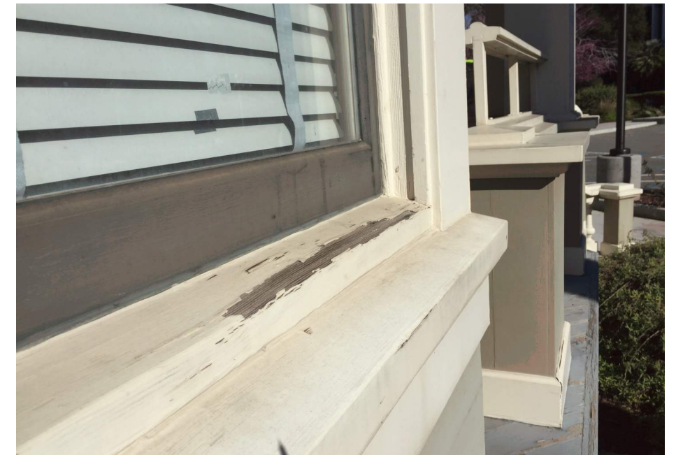
Sill and window joint deterioration, 2017 (Page & Turnbull)
