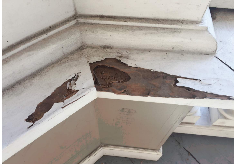
Insect damage in porch railing, 2017 (Page & Turnbull)
