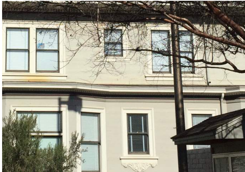
Yellow haze on exterior and deteriorated boards on second level, 2017 (Page & Turnbull)
