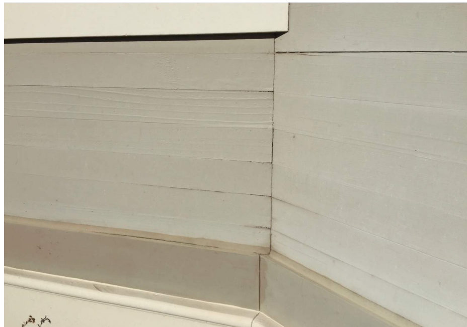
Typical deterioration of exterior boards at west facade due to sun exposure, 2017 (Page & Turnbull)
