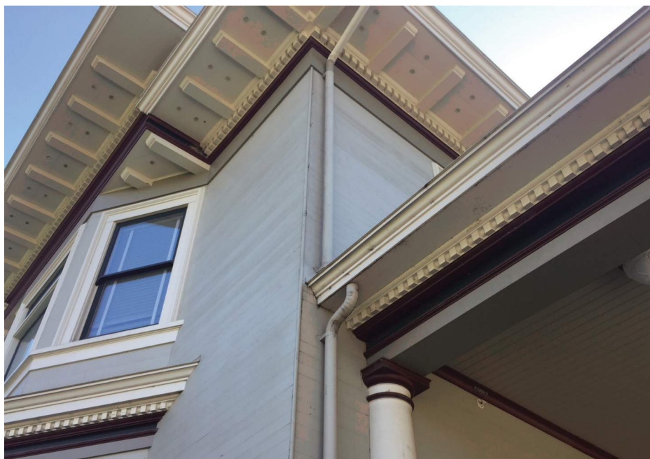
Possible deterioration of the exterior boards above the north porch , 2017 (Page & Turnbull)
